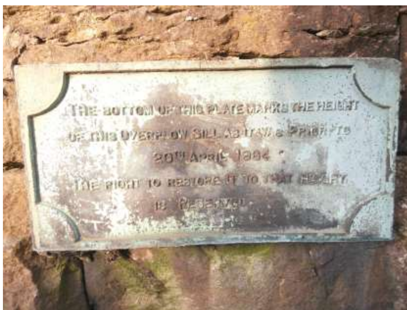
The bottom of this plaque marks the height of this overflow sill as it was prior to the 20th April 1934 the right to restore it to this height is reserved
